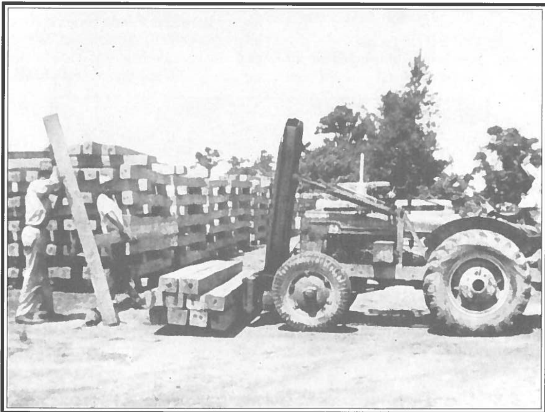
Two Ways For the "Common" Laborer To Get the Bottom Ties Onto the Lift Are Shown In This Picture. Since This Stack Was On Blocks Instead of Culls, the Last Load Has 12 Ties.
