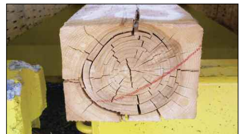
This clear example of "shake" would prevent this tie from ever being used in mainline track. Can you tell from the picture what species this is? Well, RTA tie grading seminar graduates can!
