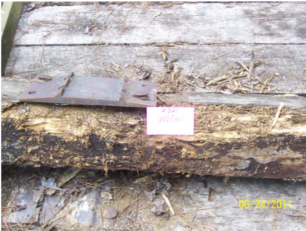
Figure 7 - Tie #321 (white oak/untreated) with extensive decay found at the time of inspection.
