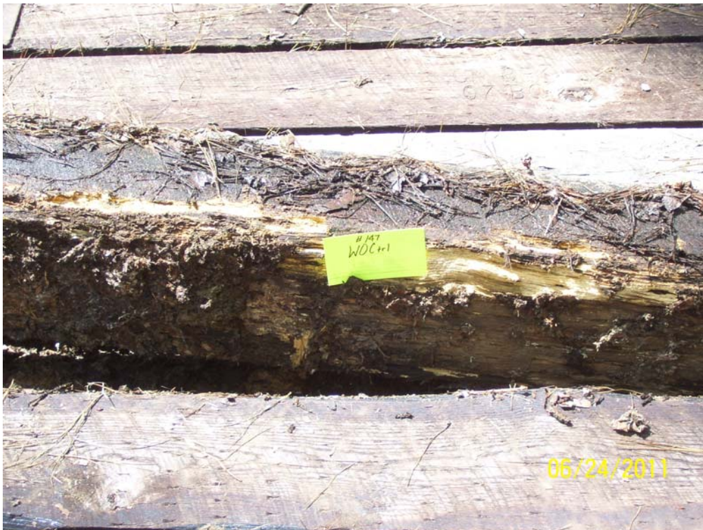
Figure 5 - Tie #147 (white oak/untreated) showing signs of obvious decay.
