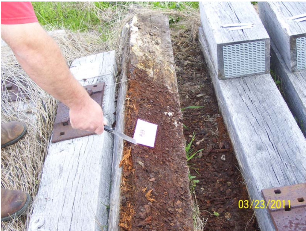
Figure 11 - #83 showing signs of decay upon inspection of lower face.
