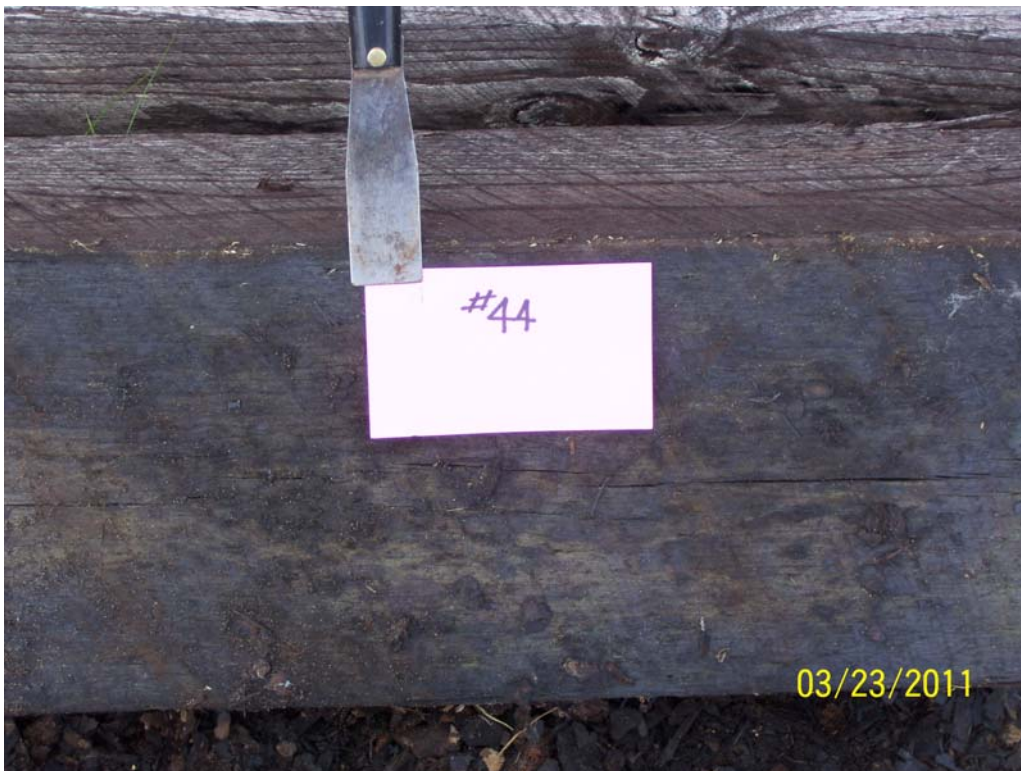
Figure 9 - Tie #44 Very clean and no signs of problems at time of inspection.
