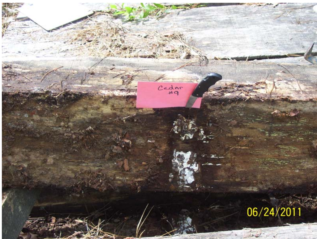
Figure 3 - Tie #9 showing decay.
