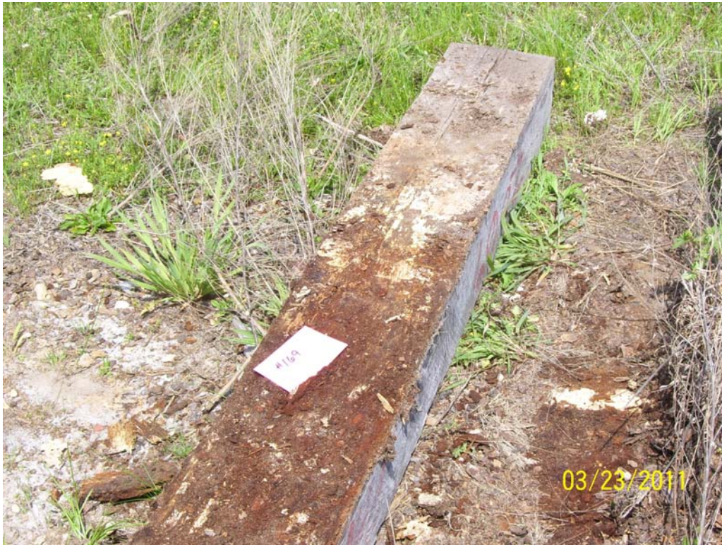
Figure 10 - #169 active decay at time of inspection.
