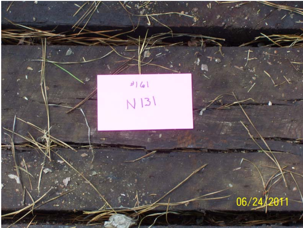
Figure 6 - Tie #161 with noticeable checking.
