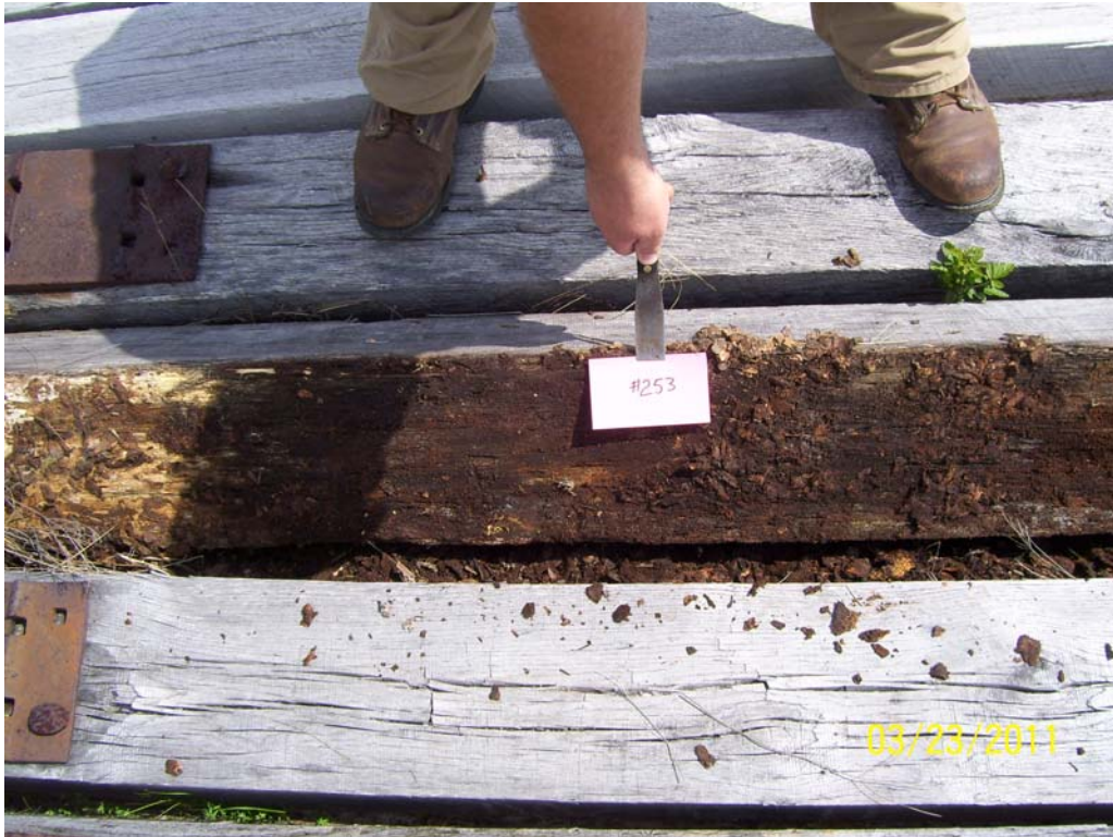
Figure 12 - #253 with signs of decay and slight termite damage visible at the time of inspection.
