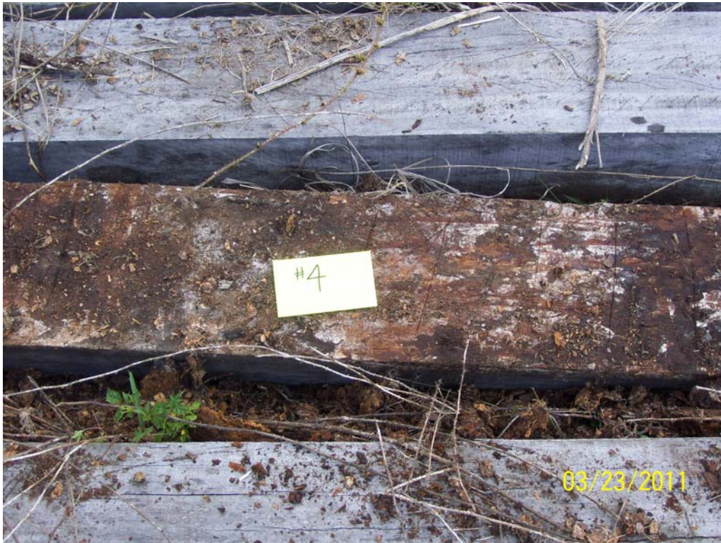
Figure 8 - Tie #4 (Turada) with light decay.
