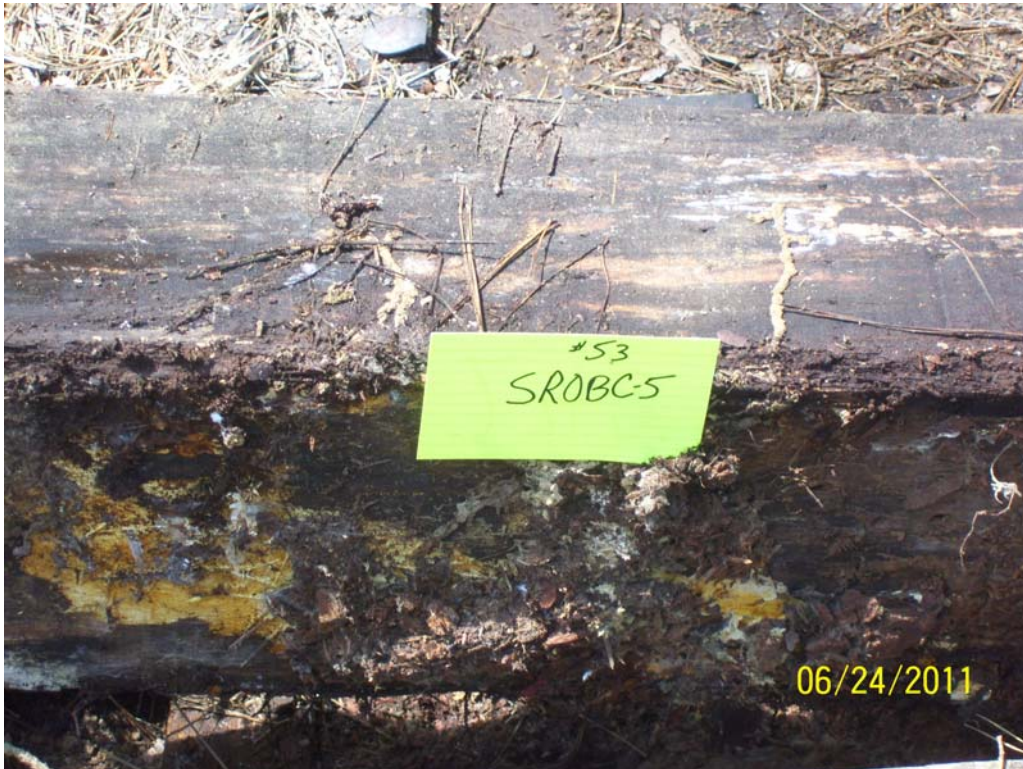
Figure 4 - Tie #53 with signs of decay and termite activity.
