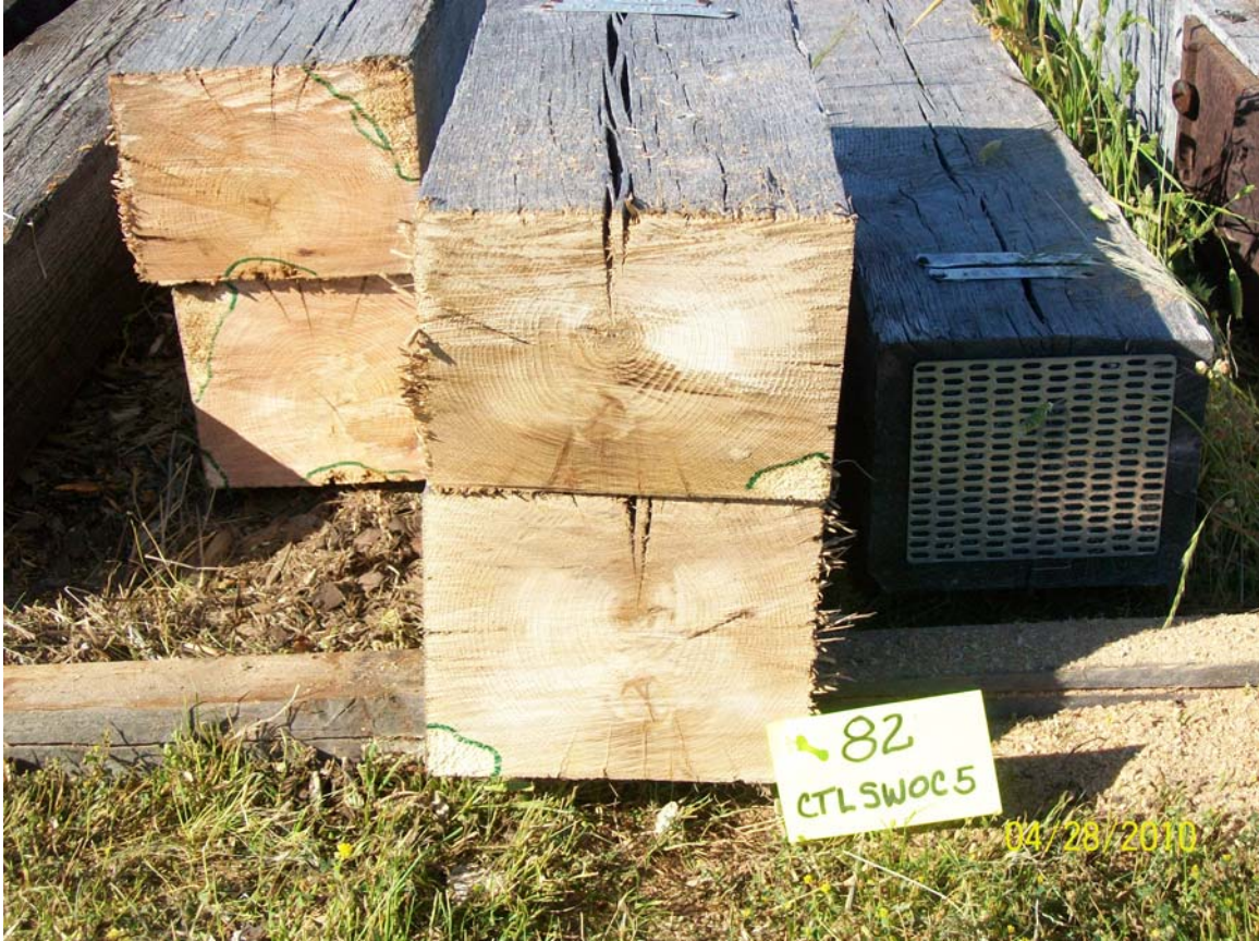
Figure 19 - Tie #82 (white oak/untreated) with decayed areas outlined.
