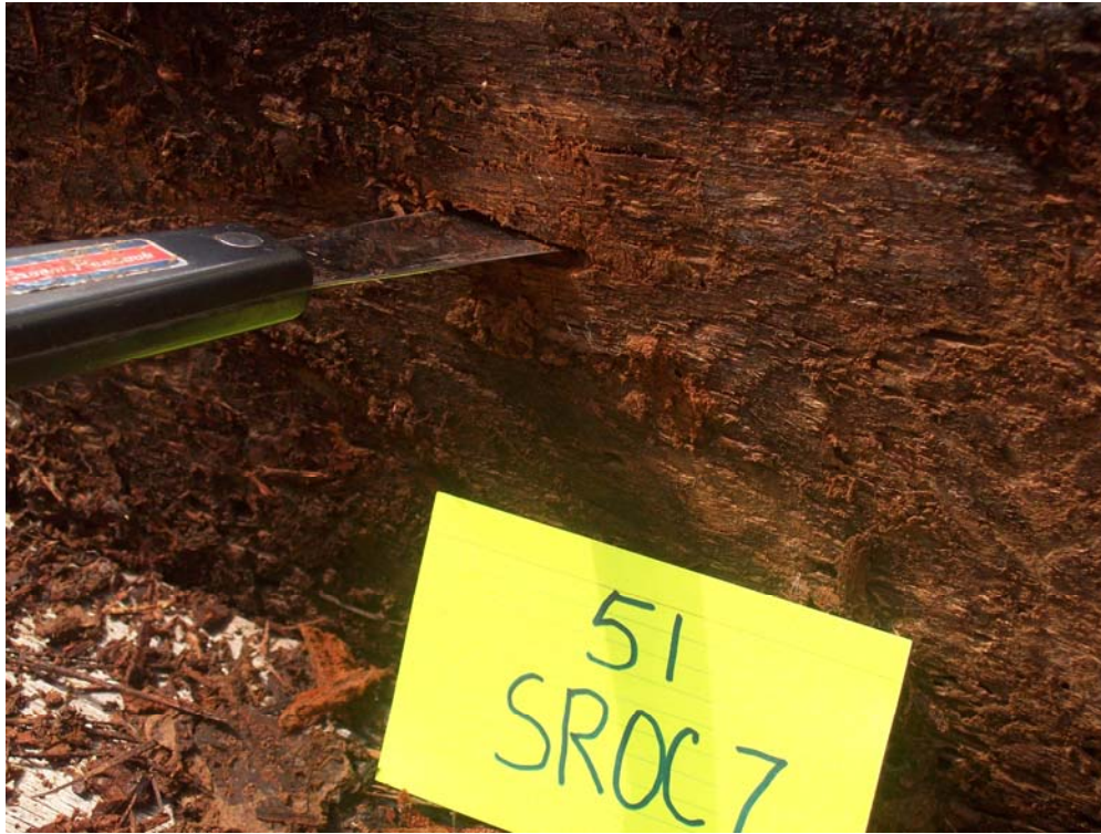
Figure 6 - Tie #51 (red oak/untreated) with penetrating decay pocket.
