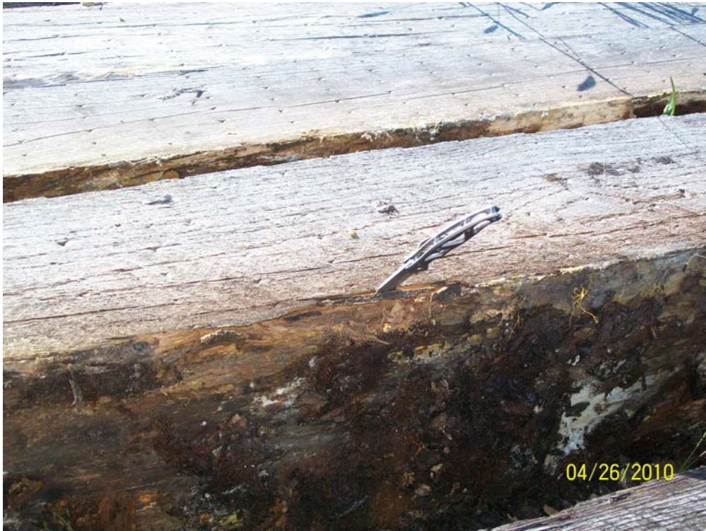
Figure 10 - Untreated tie with decay.
