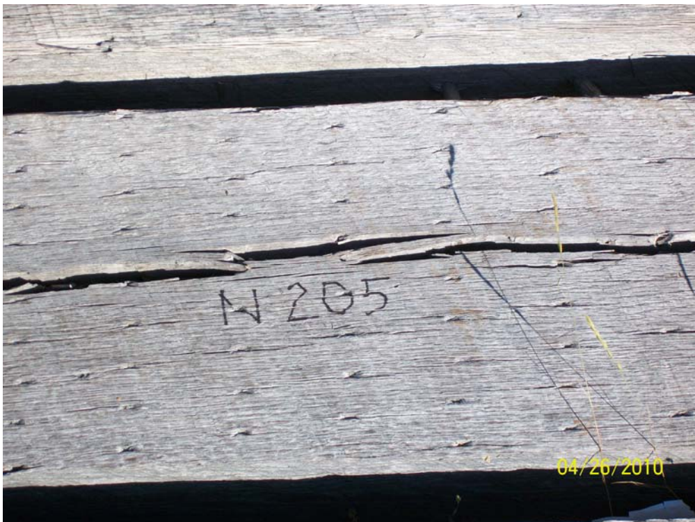
Figure 9 - Tie #130 (Nisus/red oak/borate only) with checking.
