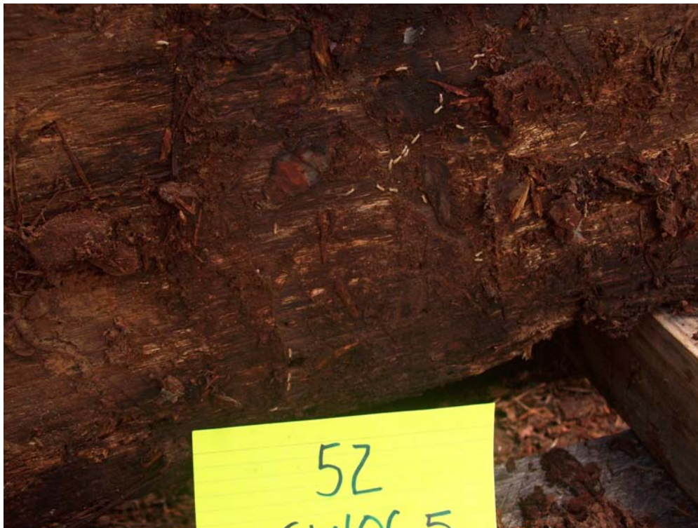
Figure 7 - Tie #52 (white oak/untreated) with live termites at the time of inspection.
