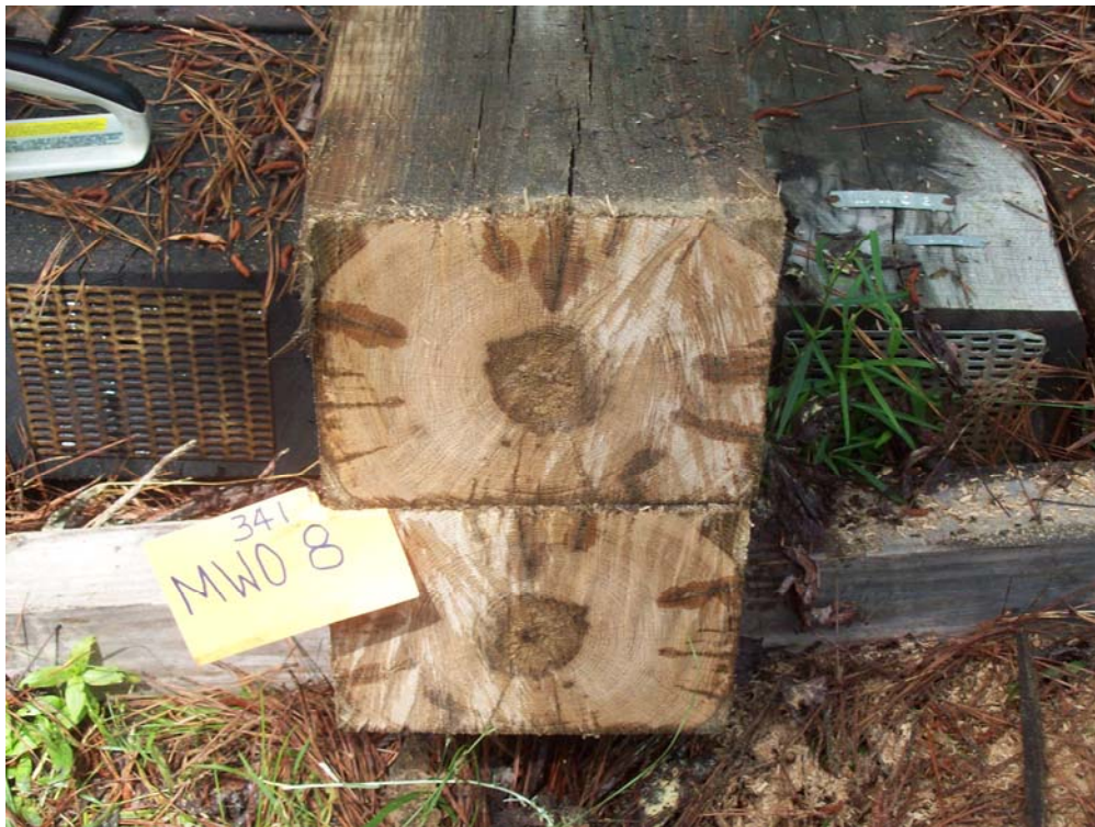
Figure 2 – Tie #341 (Merichem/white oak/air dried/CuNap) at the time of inspection contained suspected pretreatment heart rot.
