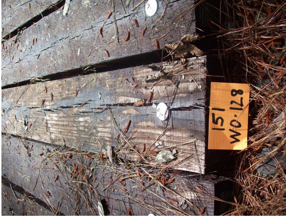
Figure 4 - Tie #151 (Nisus/white oak/borate/oil B) with heavy checking.
