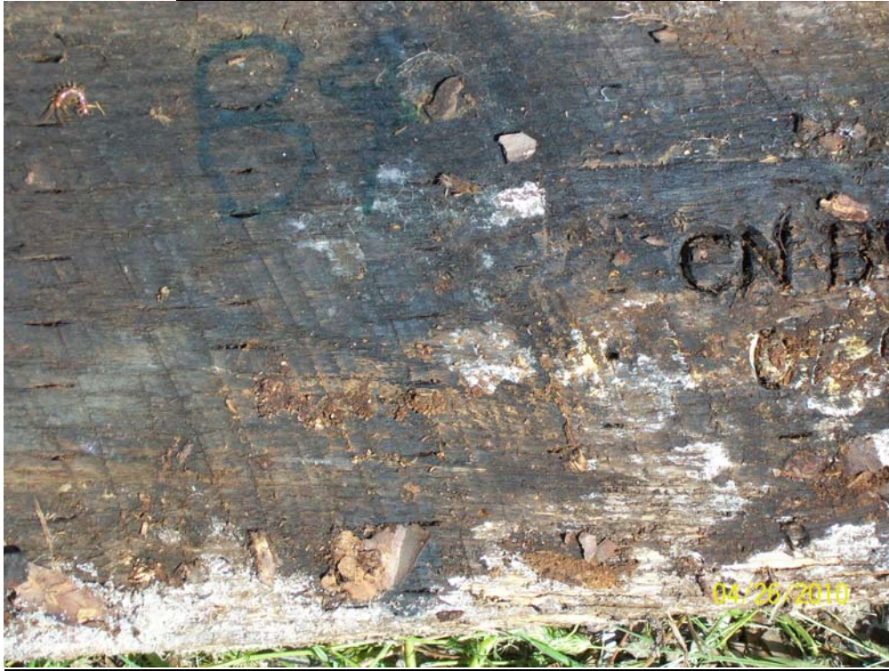
Figure 8 - Tie #84 (Lonza/red oak) with light decay.
