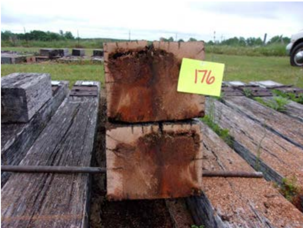
A104 - Tie #176 (Lonza/red oak) with decay.
