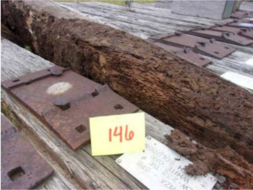
A93 - Tie #146 (Lonza/white oak) with decay and active Formosan termites.
