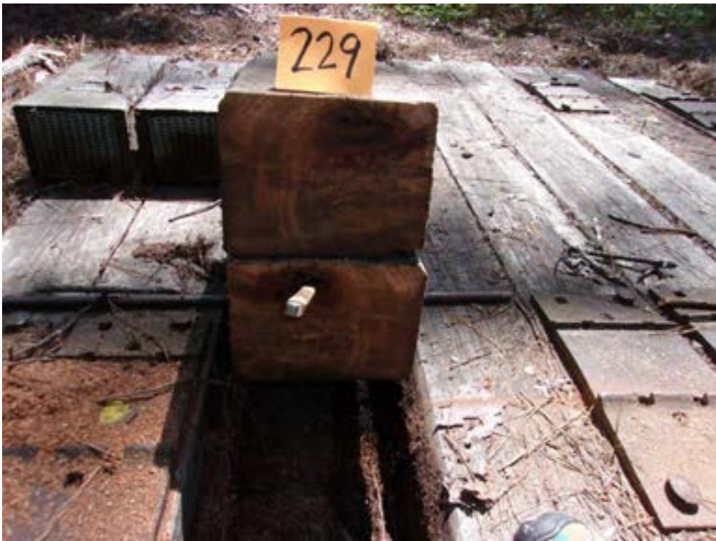
A48 - Tie #229 (Merichem/red oak/CuNap) with internal decay.
