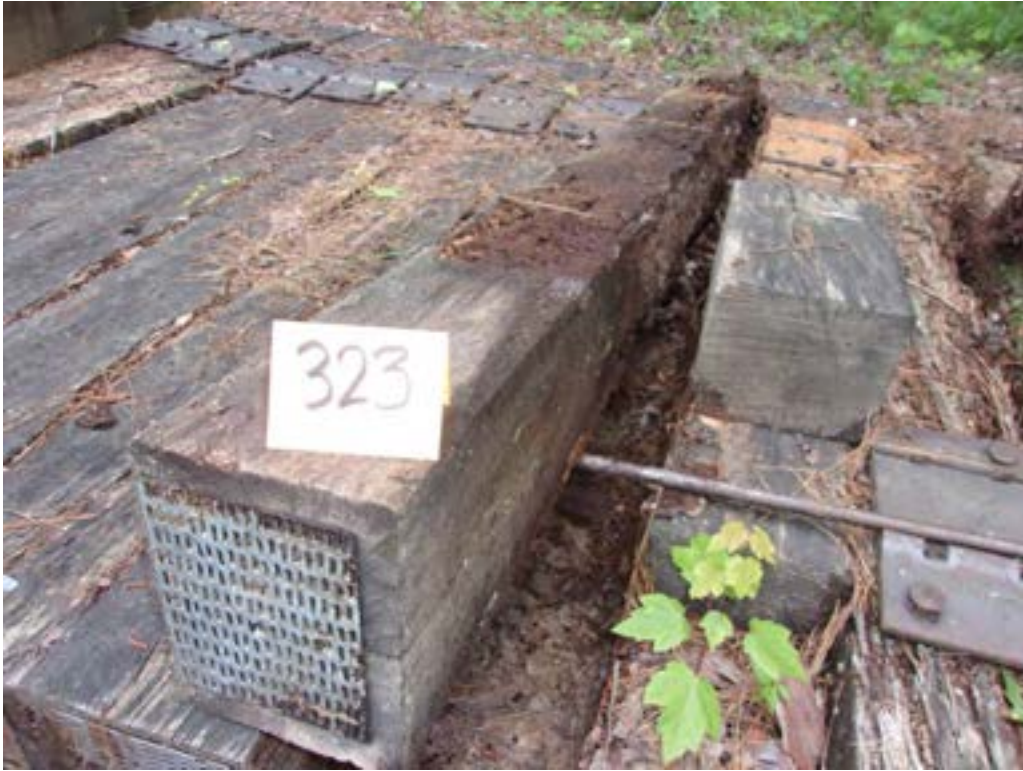
A63 - Tie #323 (Envirosafe/white oak) with decay on bottom.
