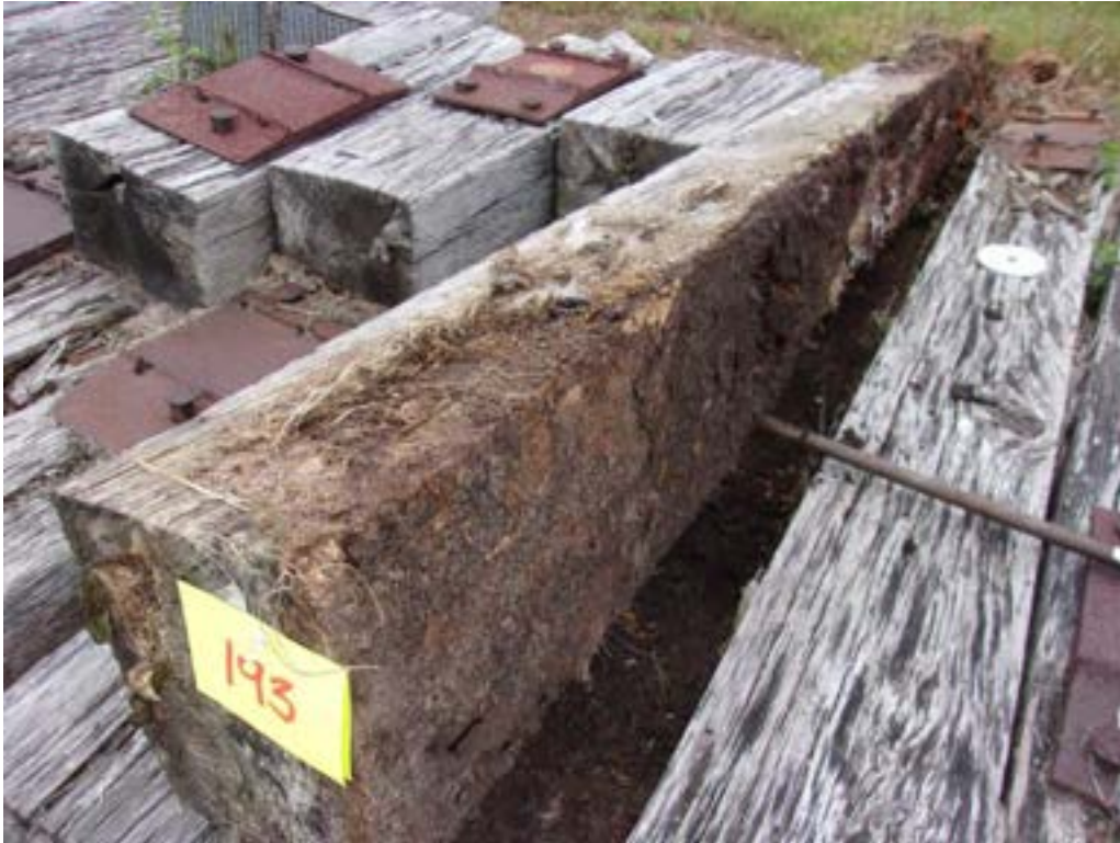
A105 - Tie #193 (Cedarcide/white oak) decay & termite damage.
