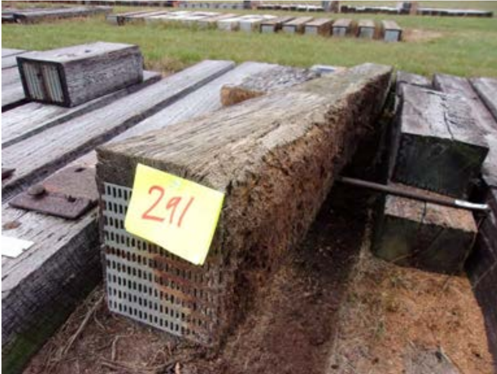
A97 - Tie #291 (untreated/red oak) with decay
