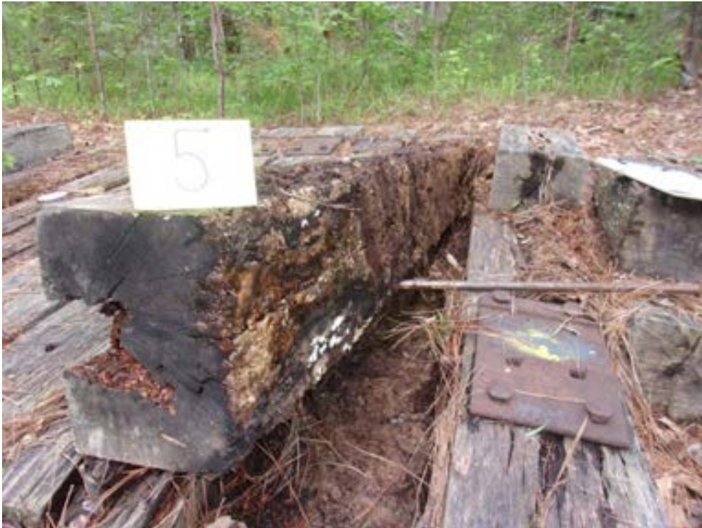
A1 - Tie #5 (Cedarcide/white oak) with extensive decay.
