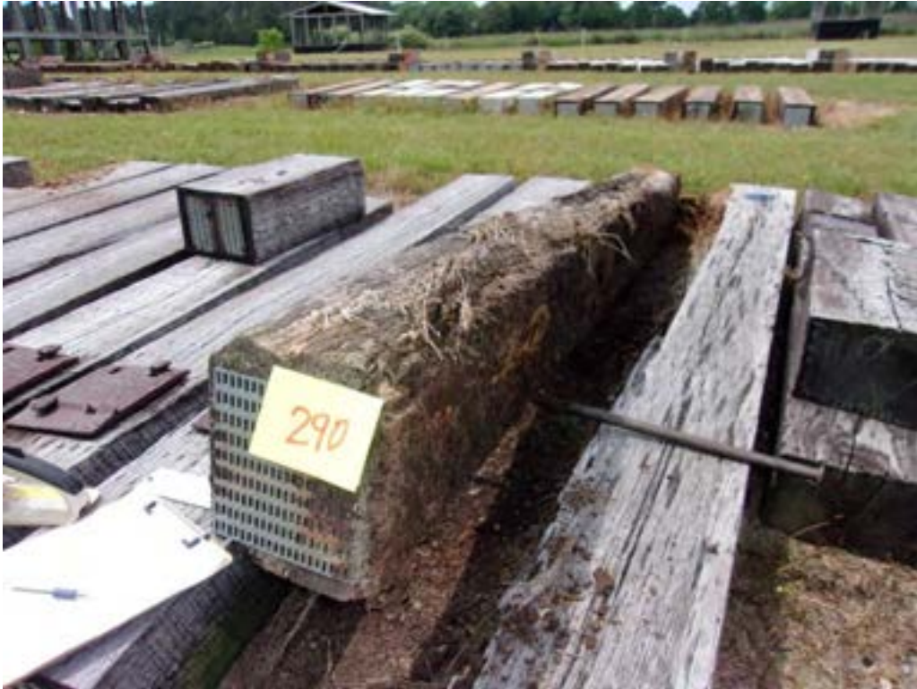
A95 - Tie #290 (untreated/White oak) with heavy decay.
