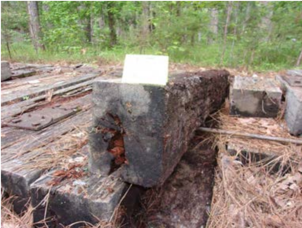
A3 – Tie #15 (Cedarcide/red oak) with decay.
