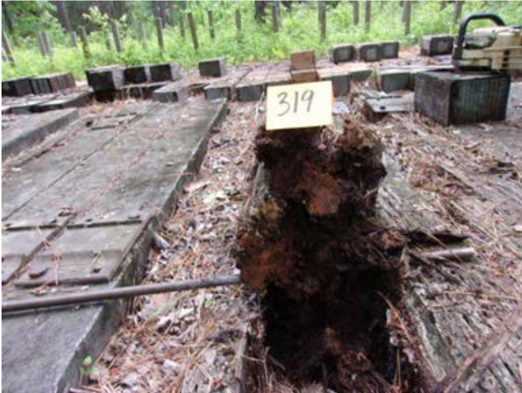
A29 - Tie #319 (untreated/red oak) completely deteriorated.
