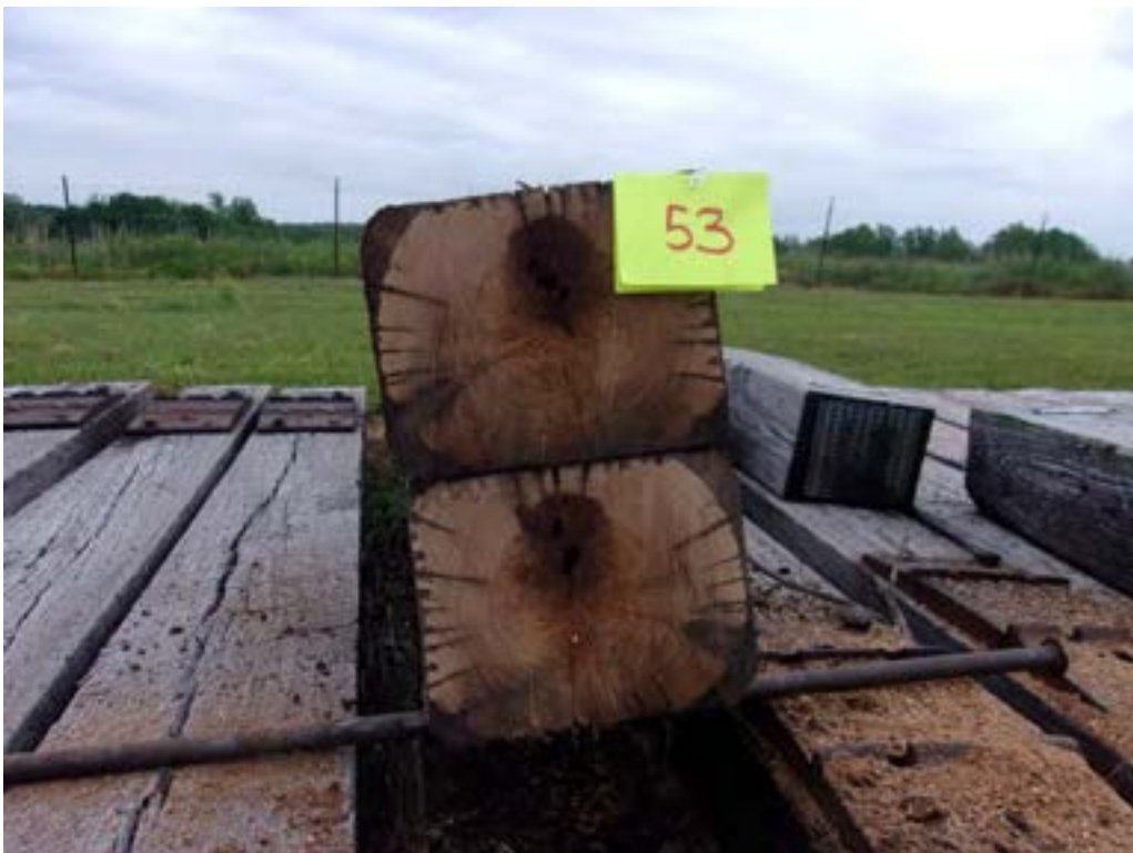
A76 - Tie #53 (Boatright/white oak//creosote to refusal) with internal decay.
