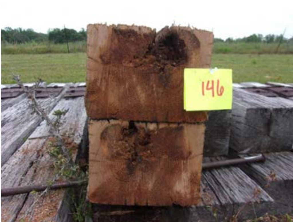
A94 - Tie #146 (Lonza/white oak) with internal decay.
