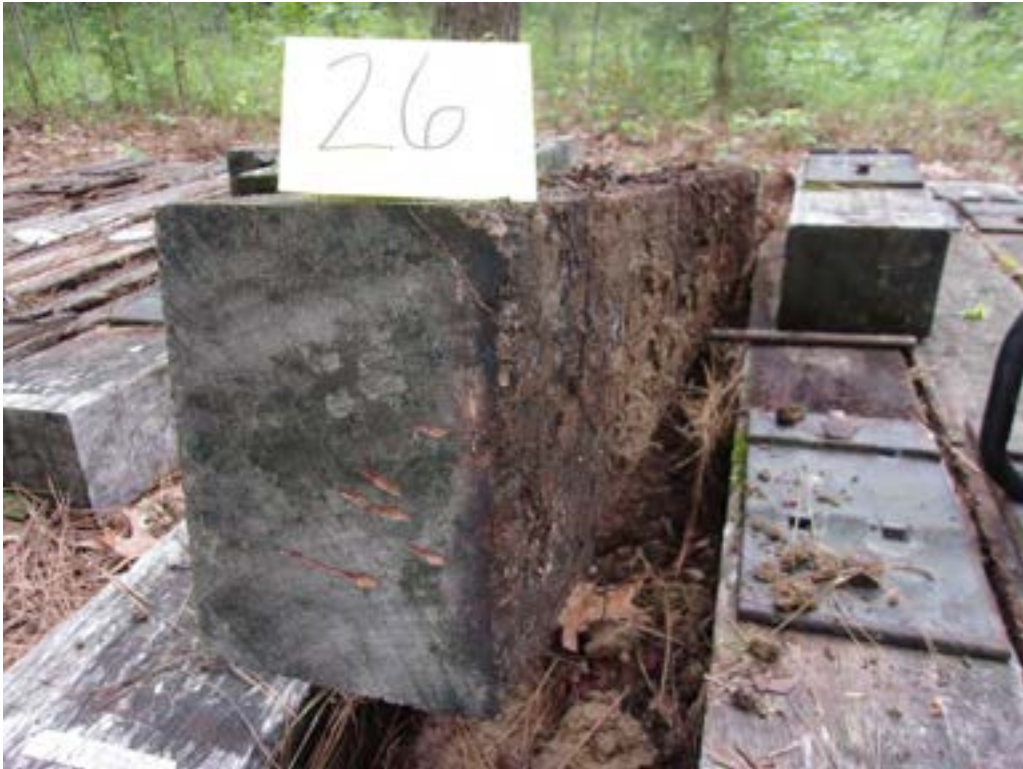
A5 – Tie #26 (Turada) with decay on bottom and side.
