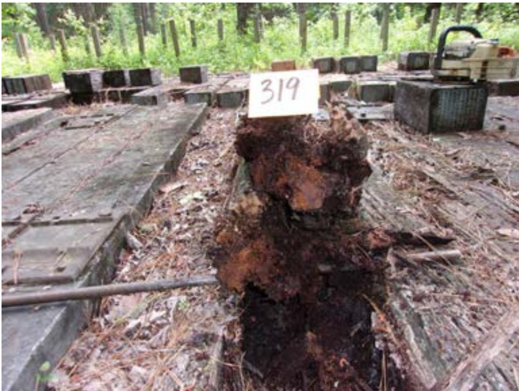
A30 - Tie #319 (untreated/red oak - closer view of failed tie/decay).
