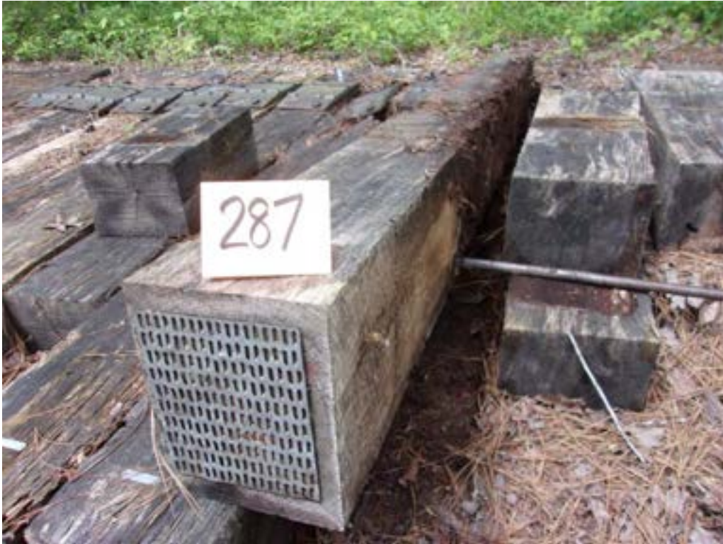
A61 - Tie #287 (Envirosafe/red oak) with decay on bottom.
