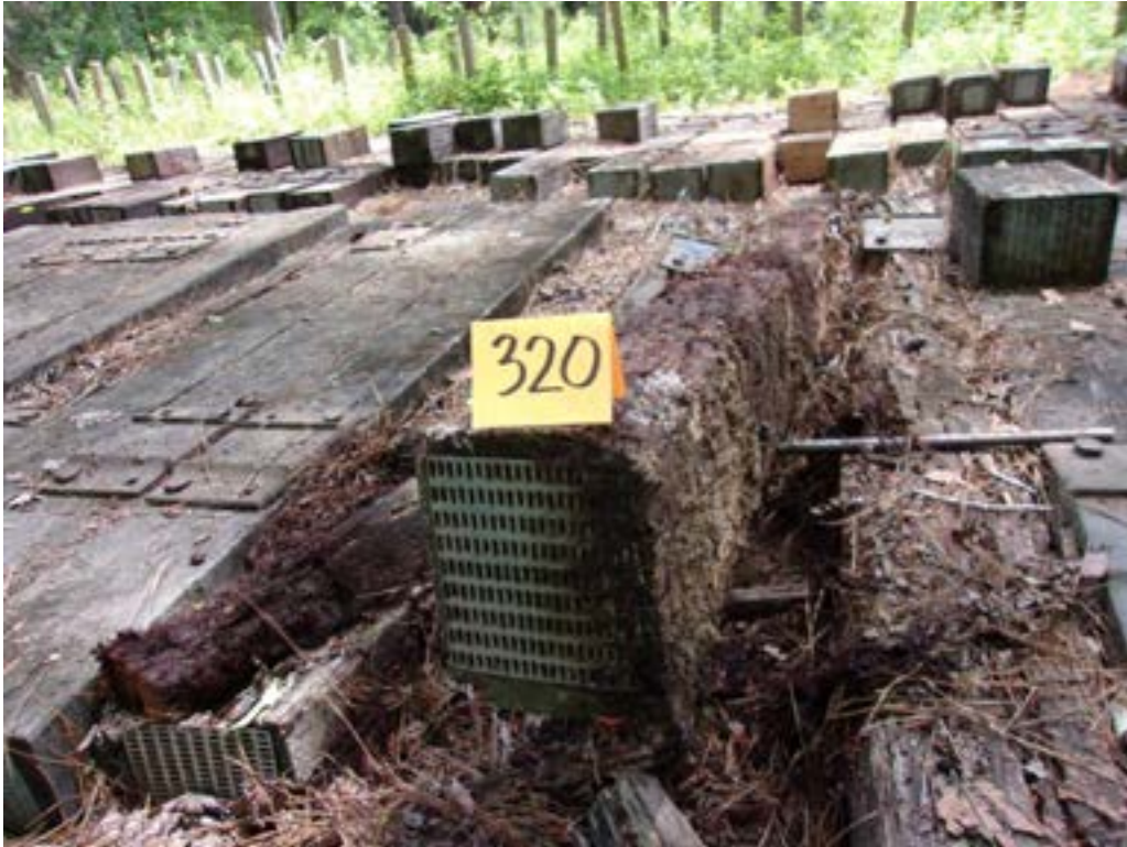
A45 - Tie #320 (untreated/white oak) with decay.
