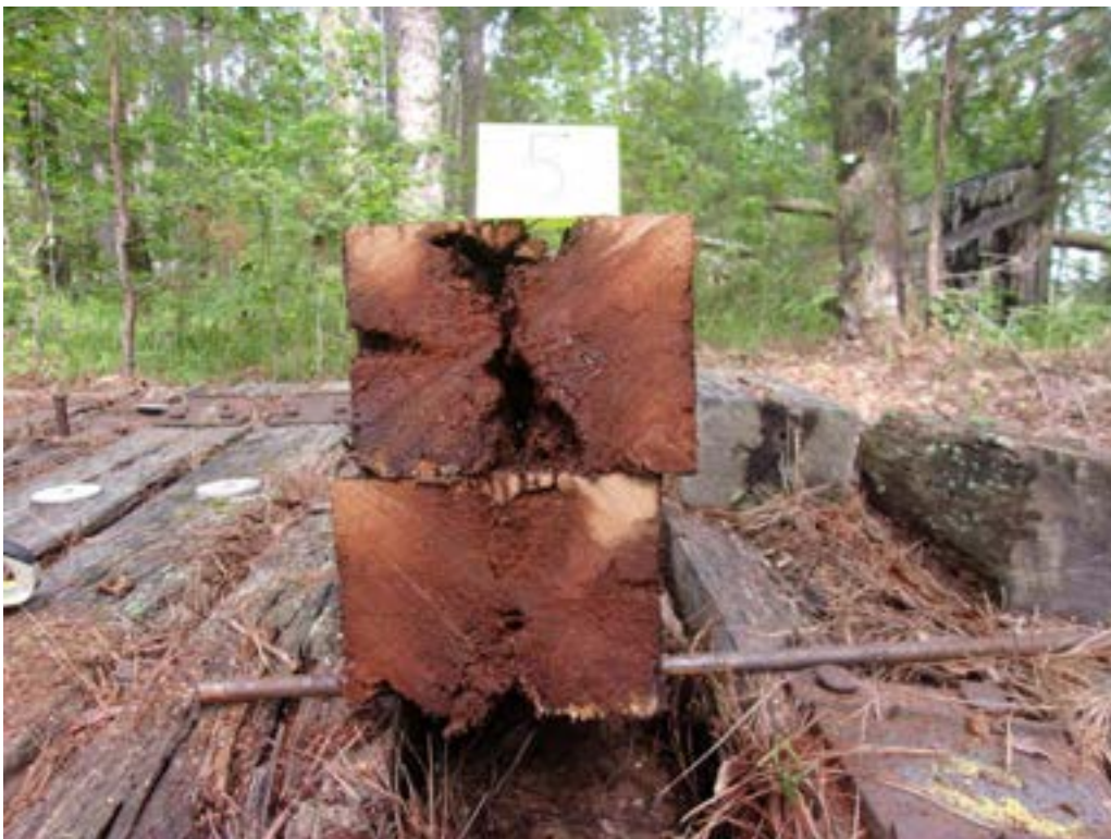
A2 - Tie #5 (Cedarcide/white oak) with extensive decay.
