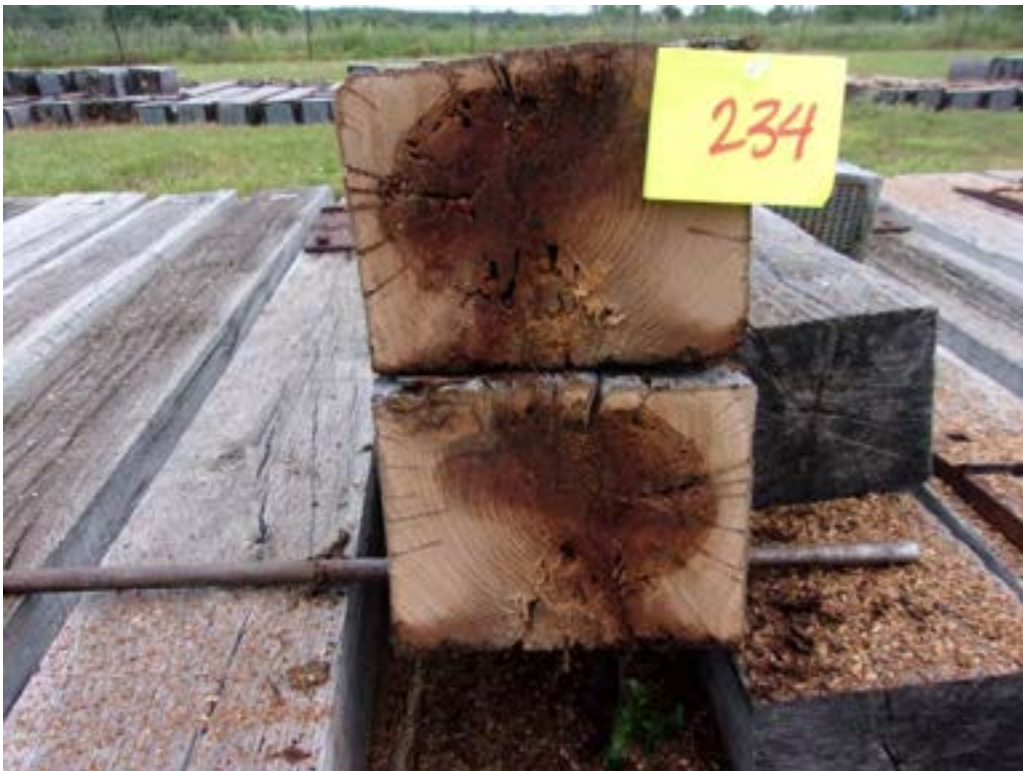
A114 - Tie #234 (Merichem/white oak/CuNap) with decay & Formosan termites.
