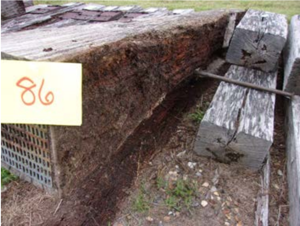
A81 - Tie #86 (Lonza/red oak) decay on bottom.
