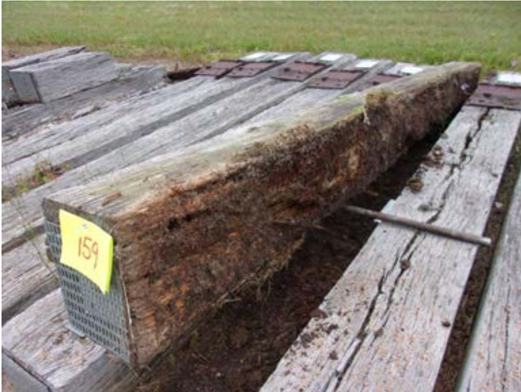
A101 - Tie #159 (Nisus/white oak/boron) with decay on bottom.
