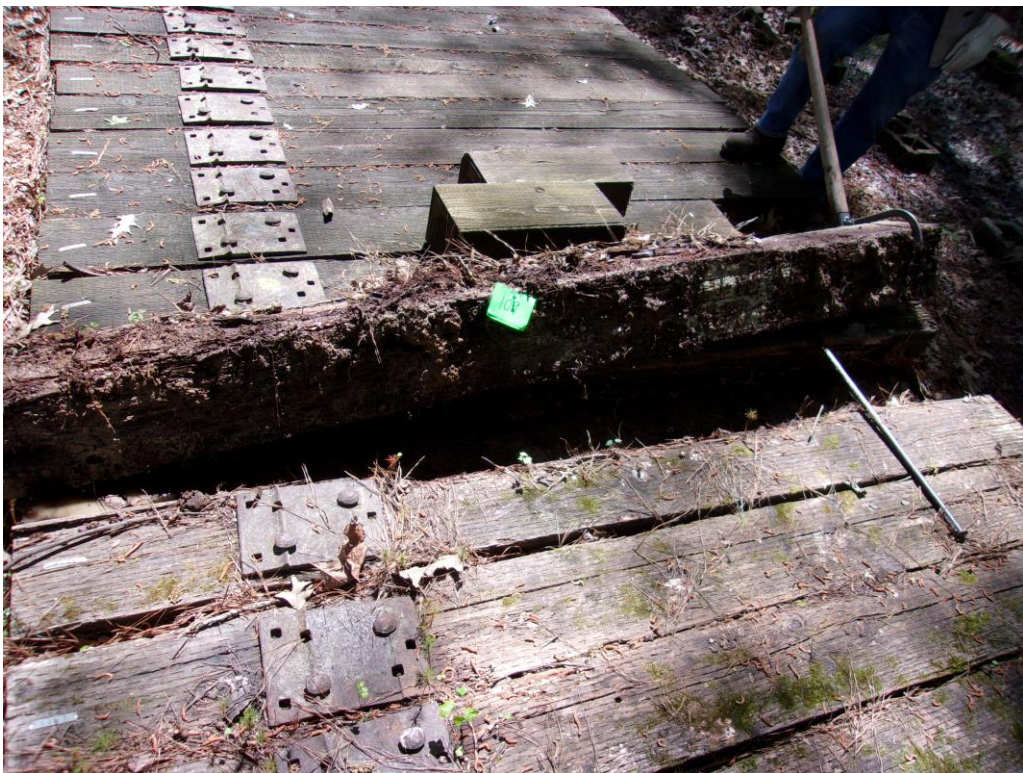
Figure 5 - Tie 109 with decay.
