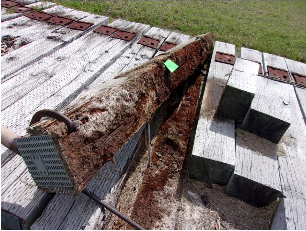
Figure 8 - Tie 110 with decay and light Formosan termite damage.
