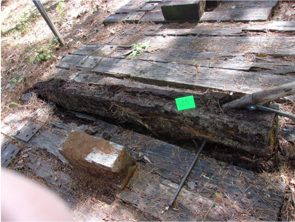
Figure 2 - Tie 25 showing signs of severe deterioration
