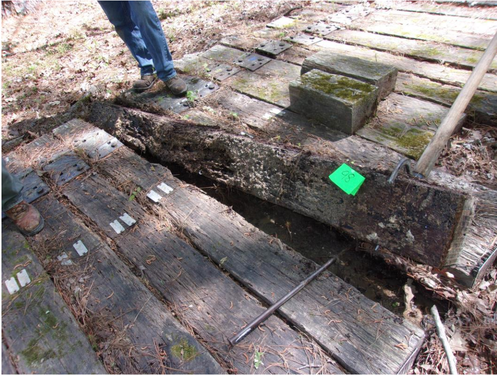
Figure 4 - Tie 70 with decay and light termite damage.
