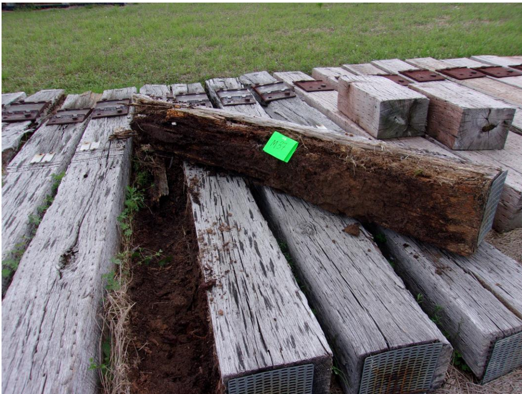
Figure 7 – Tie 37 which failed from decay and also had termite damage.
