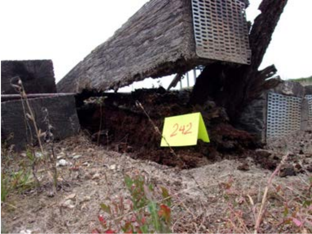
Figure 103 – Tie #242 untreated red oak with heavy decay and Formosan termites.
