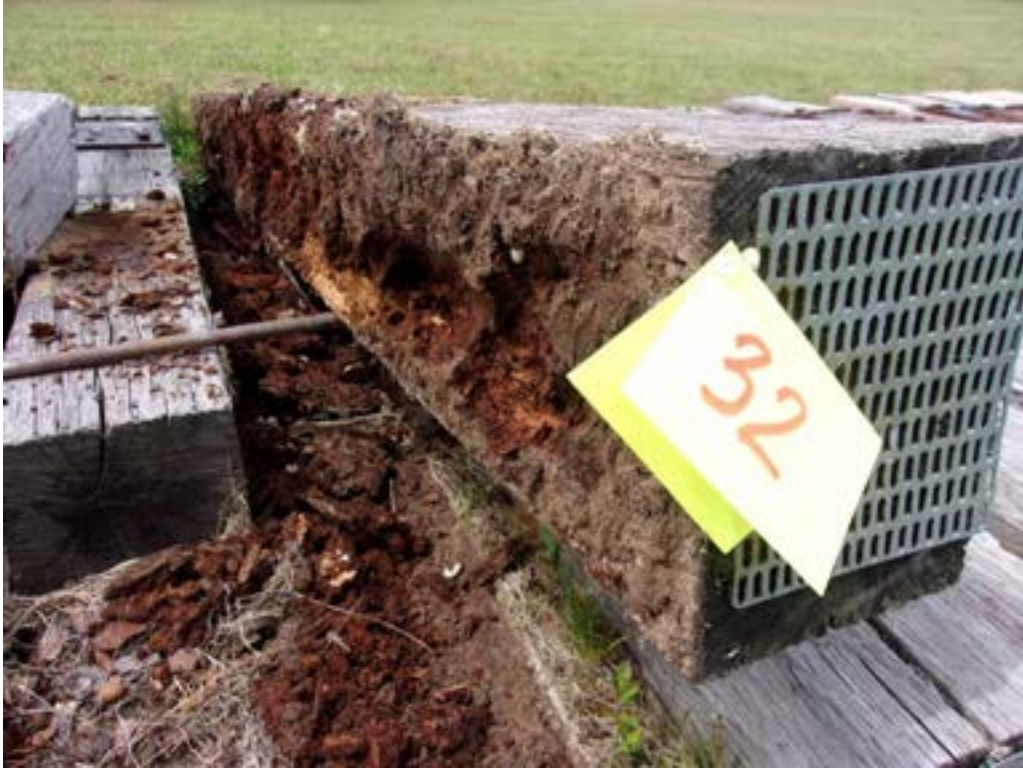
Figure 59 – Tie #32 untreated white oak with decay and beetle damage.
