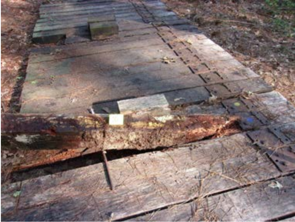
Figure 5 – Tie #22 failed untreated red oak with heavy decay and termite damage.
