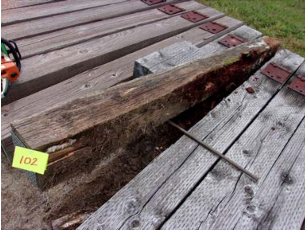
Figure 73 – Tie #102 untreated Douglas fir with decay.
