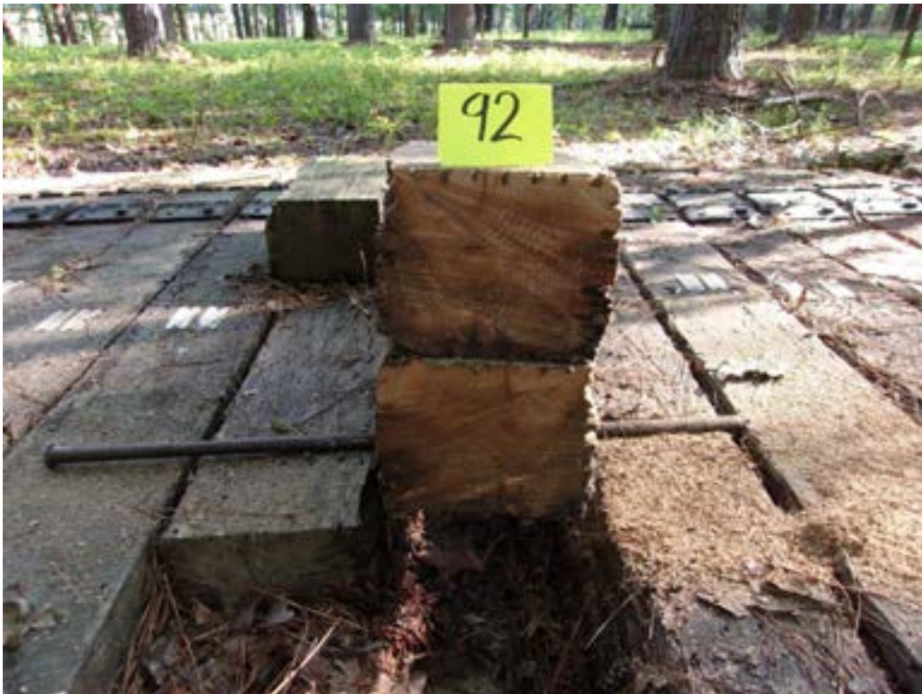
Figure 20 – Tie #92 untreated white oak with decay visible.
