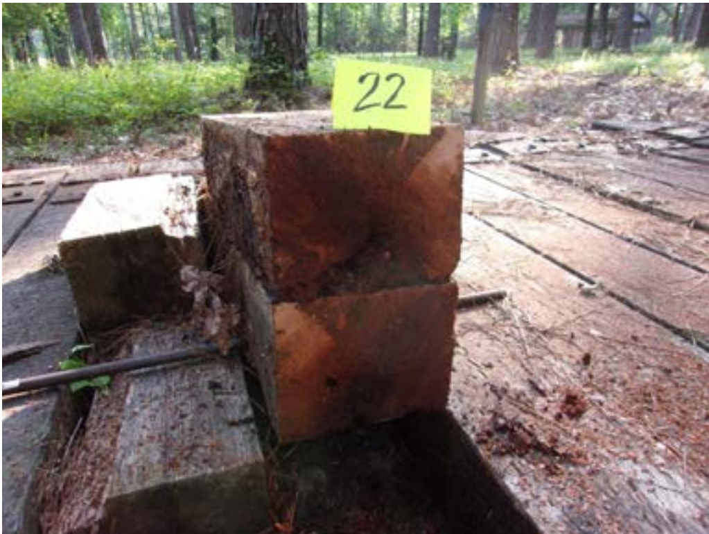
Figure 6 – Tie #22 untreated red oak with extensive decay.
