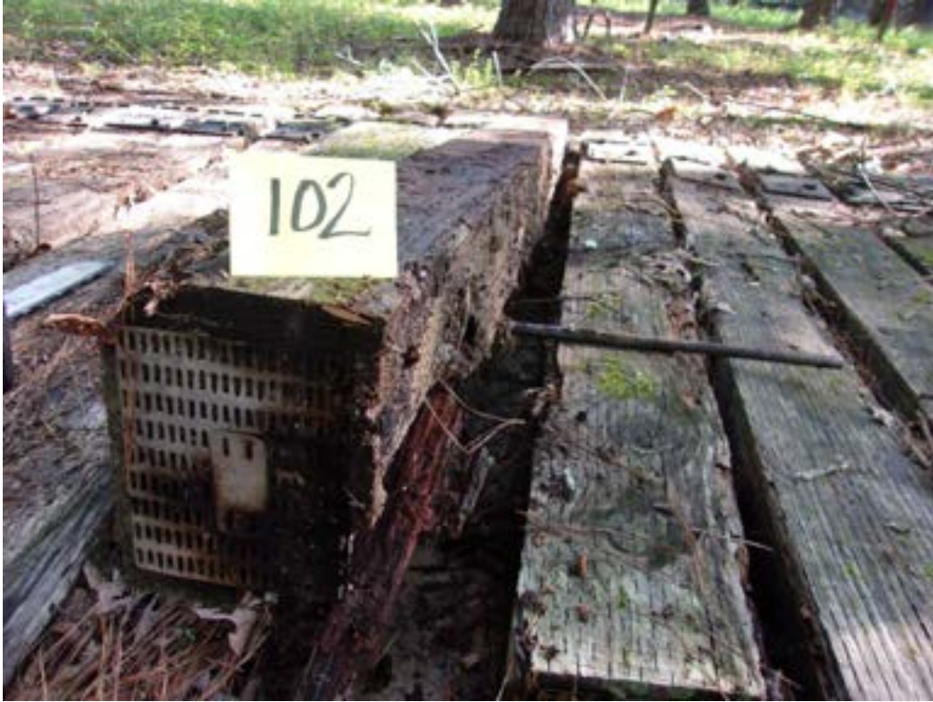
Figure 21 – Tie #102 untreated Douglas fir with decay and active termites ( Reticulitermes ).
