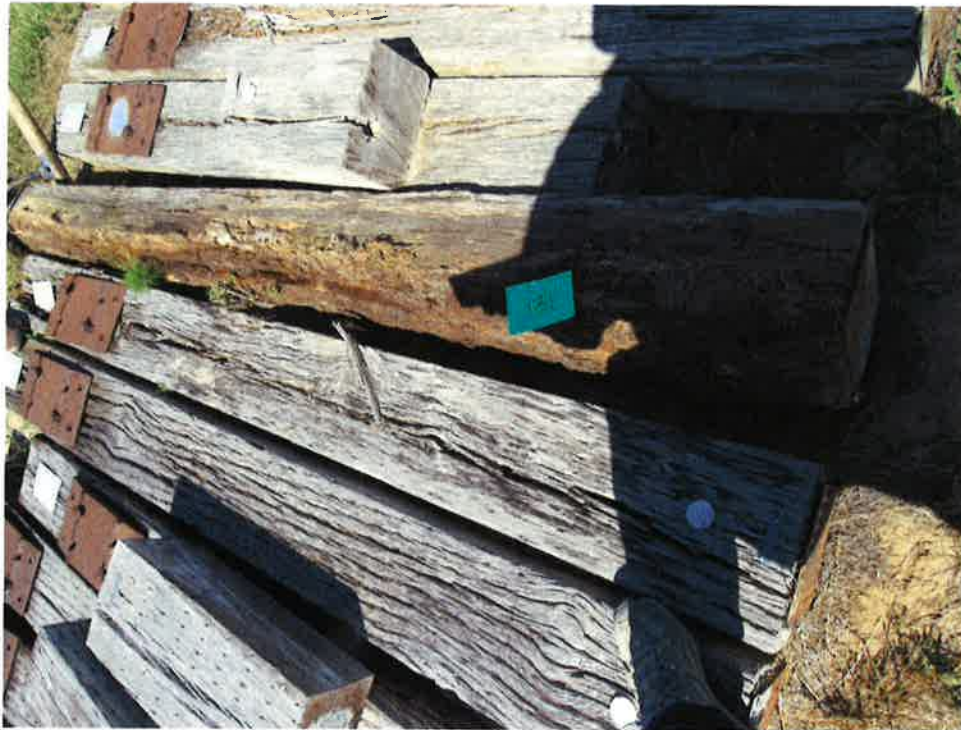
Figure 6 - Tie #131 with extensive decay.
