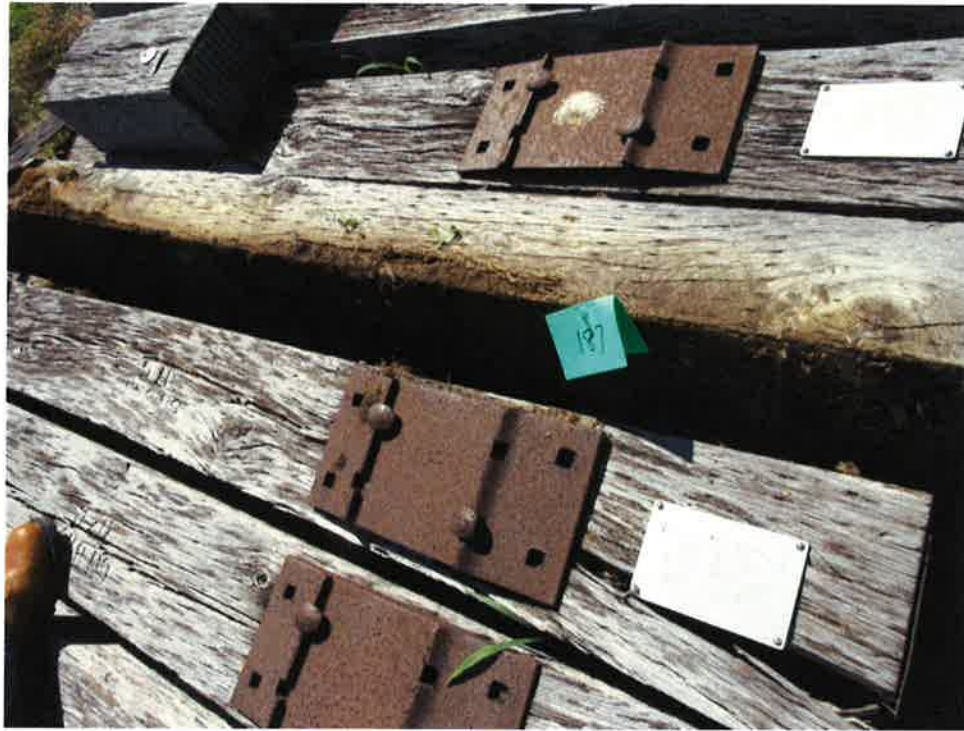
Figure 8 - Tie #187 with active Formosan subterranean termites (FST).
