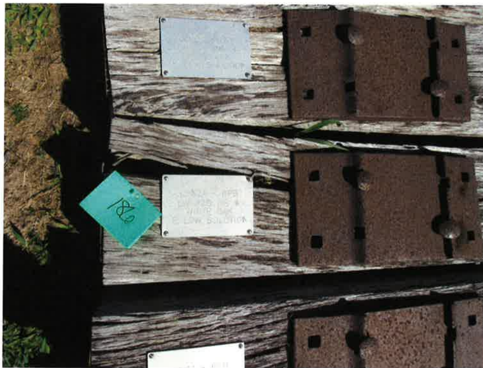
Figure 7 - Tie #186 with "alligator" end.
