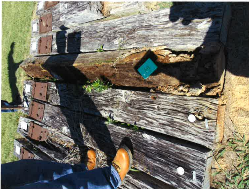
Figure 5 - Tie #89 with heavy decay and termite damage.
