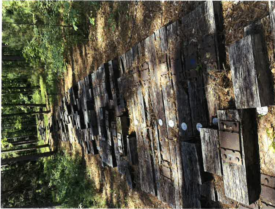
Figure 4 – Another overall view showing the abundant vegetation growth around ties due to the heavy rainfall.
