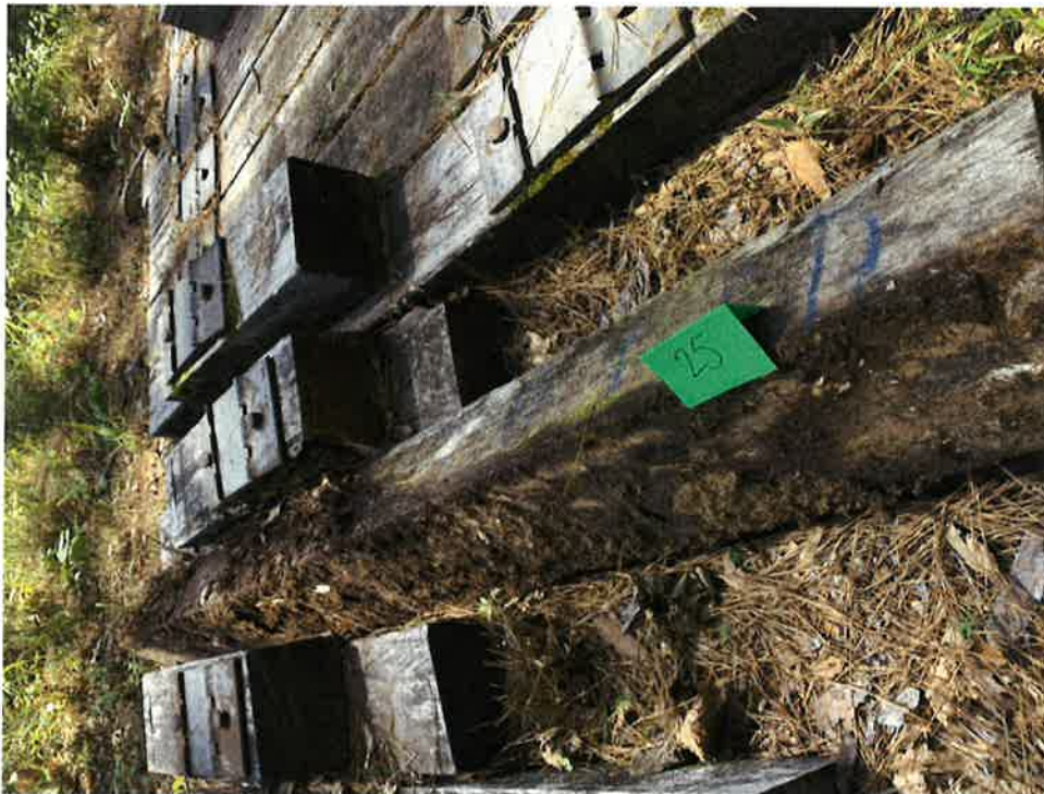
Figure 3 - Tie #25 with slight decay.
