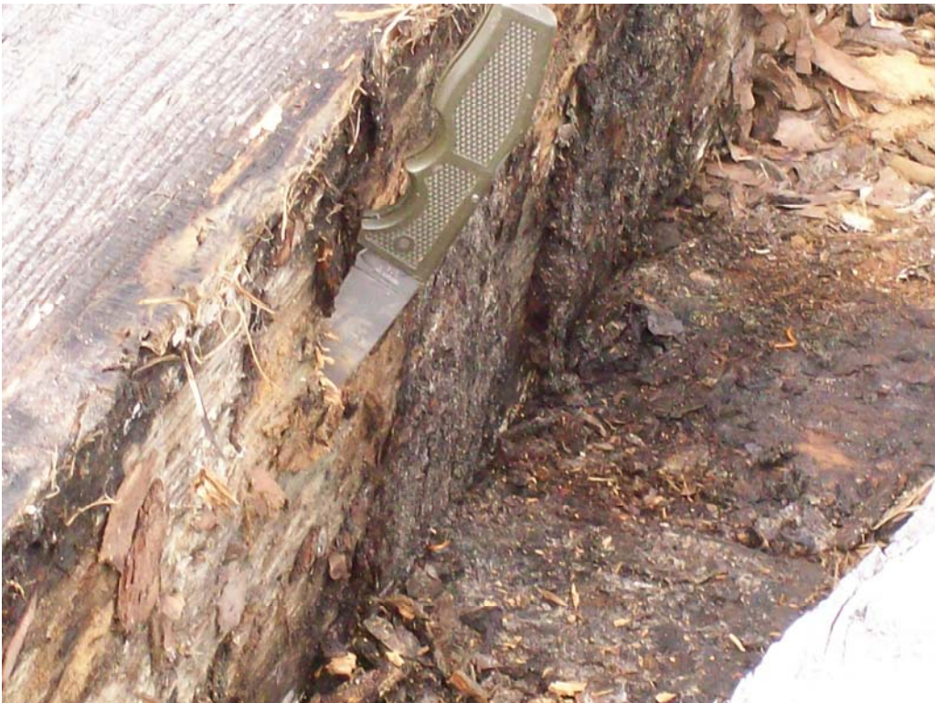
Figure 6 – Obvious decay was evident in some ties after one year of exposure (Site 1).
