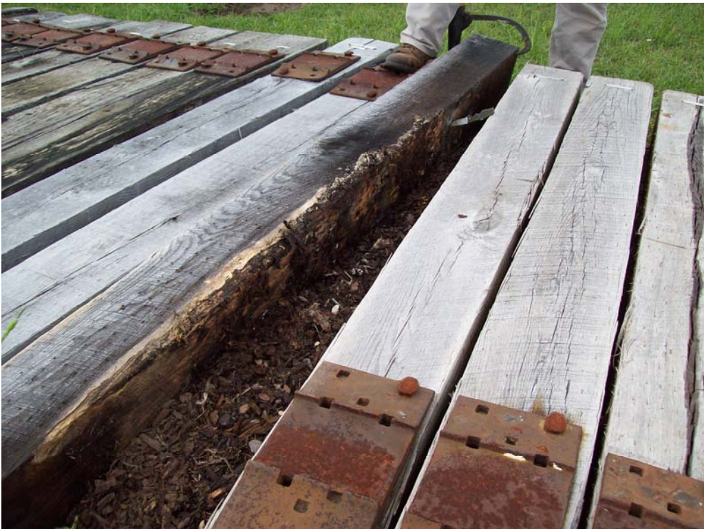
Figure 8 – After one year of exposure evidence of termite ( Coptotermes formosanus ) damage was found in some control (untreated) ties (Site 1).
