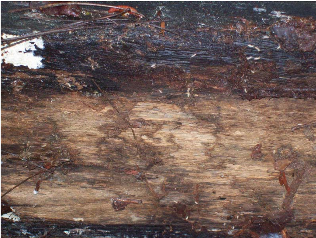
Figure 4 – After only one year of exposure, termite ( Reticulitermes flavipes ) damage was found in several control (untreated) ties (Site 2).
