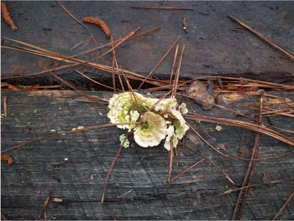
Figure 3 – Fruiting bodies of decay fungi are an obvious sign of active decay (Site 2).
