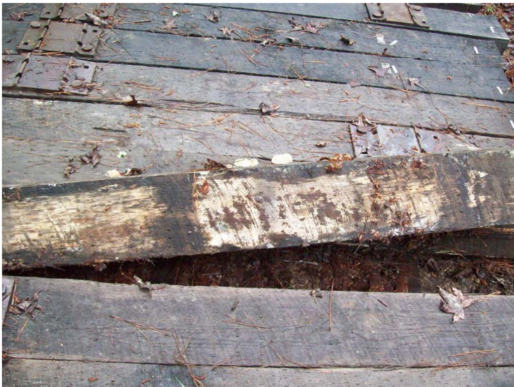
Figure 2 – After one year of exposure, evidence of decay could already be found in some ties (Site 2).
