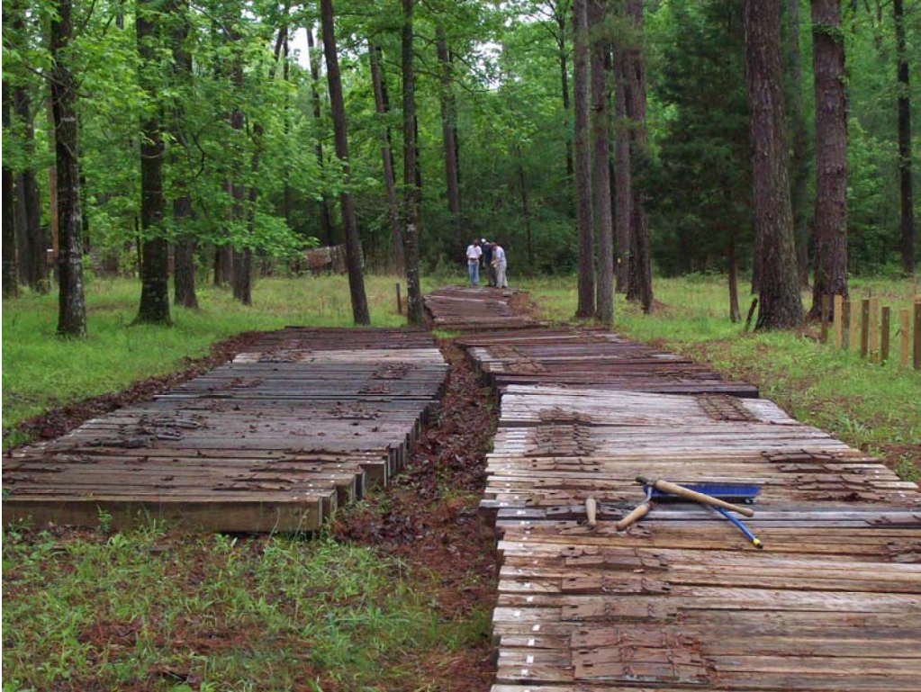
Figure 1 – An overall view of the ties exposed at the Dorman Lake research site at the time of inspection (Site 2).
