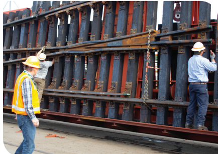
Bob Baeppler of Vance watches as workers load a completed turnout onto a rail car.
