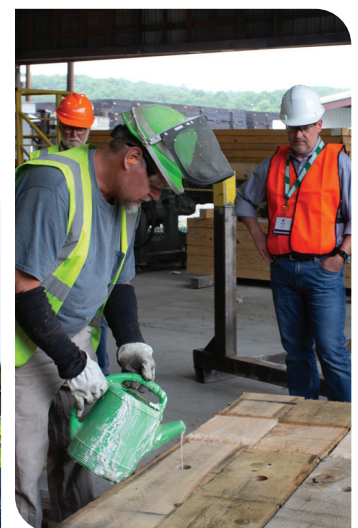
Frank Wawros of U.S. Borax and Claus Staalner of American Wood Technology watch the borate drill and fill process in bridge timbers.
