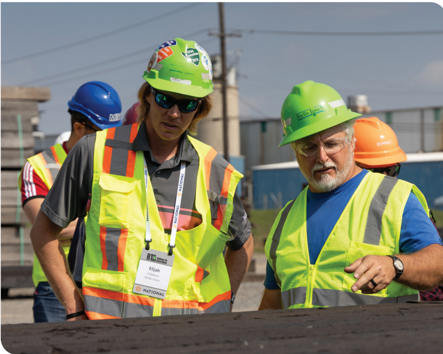
Bridge Fab Supervisor Donnie Ellis (R) explains the bridge deck process to Elijah Coleburn (L) of Stella-Jones.
