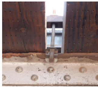
A view under the state-of-the-art bridge showing the Lewis Bolt & Nut Quick-Set® hook bolt assembly. The photo also shows the lack of dapping of the superelevated glue-laminated bridge ties. The angle of the hook bolt can be seen in the photo.
