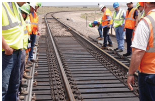
Open-deck bridge ties on the 55-foot span of the East Steel Bridge. The ties shown are a mixture of glue-laminated timber and Southern Yellow Pine. The fastener system is 8-inch-wide Progress Rail Loadmaster™ plates. The hook bolts are Lewis Bolt & Nut Quick-Set® hook bolts.
