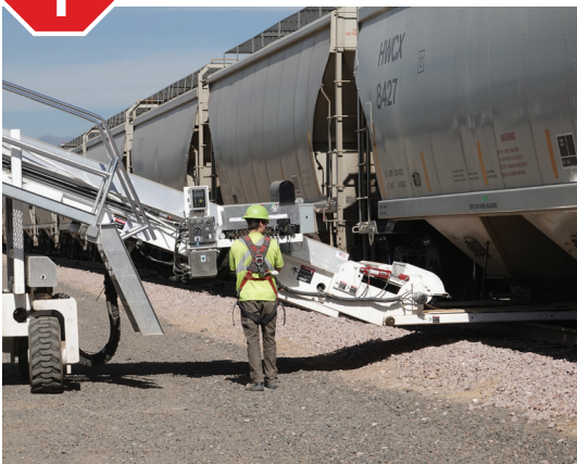
An OmniTRAX Energy Solutions employee unloads sand from railcar onto high speed conveyor for transfer to truck.
