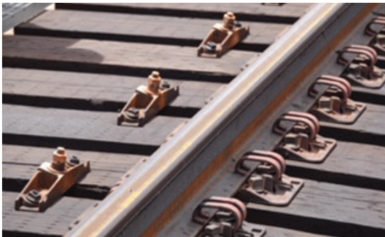
A closeup view of superelevated glue-laminated open-deck bridge ties on the state-of-the-art bridge. The ties have the superelevation built into the tie and are not dapped on the bottom. The deck uses the Lewis Bolt & Nut Quick-Set® hook bolt system to provide the active attachment of the deck to the bridge.
